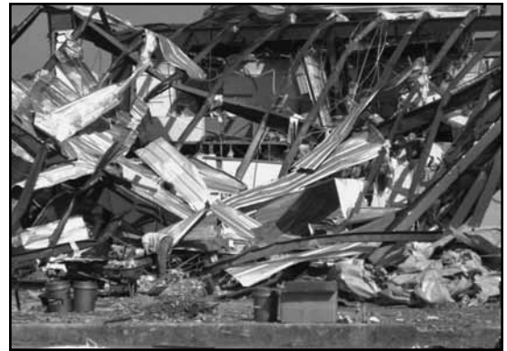
Twisted steel is evidence of the wind's power
